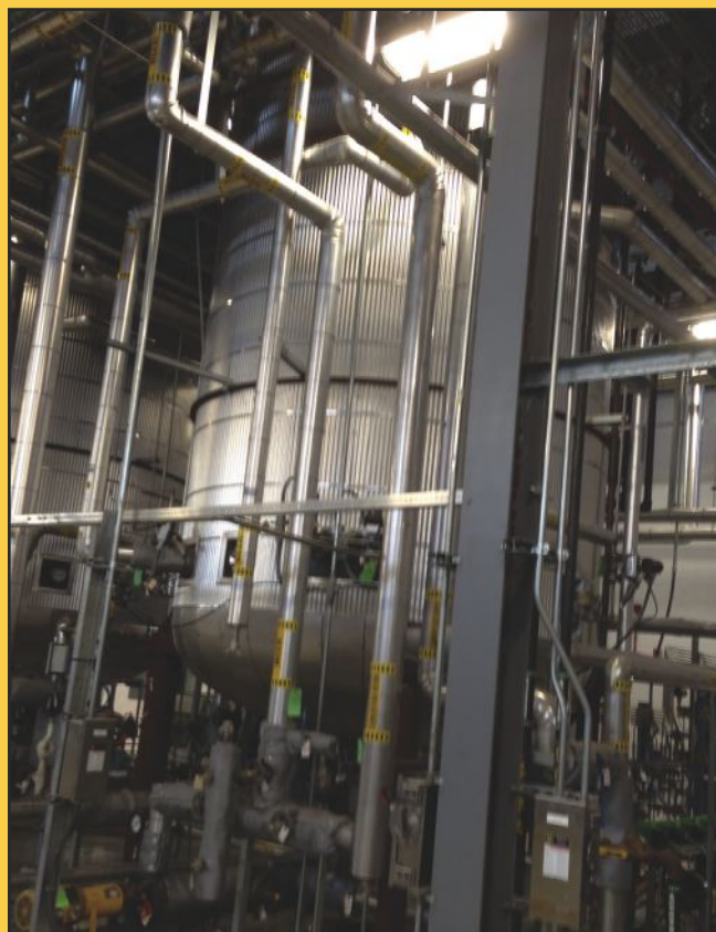
The Stan Mayfield biorefinery enables UF researchers to conduct multifaceted studies and develop economical ways to produce bioethanol and its derivatives from non-edible parts of plants and other biomass.
