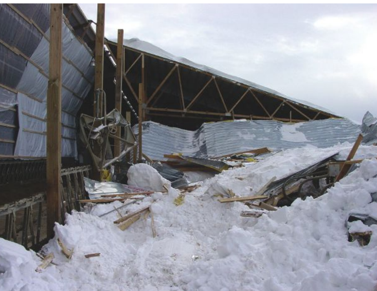
Cyril Myren and his son Todd were injured during the above roof collapse, which was attributed to a lack of diagonal bracing on the continuous lateral bracing used to keep truss web members from buckling.
