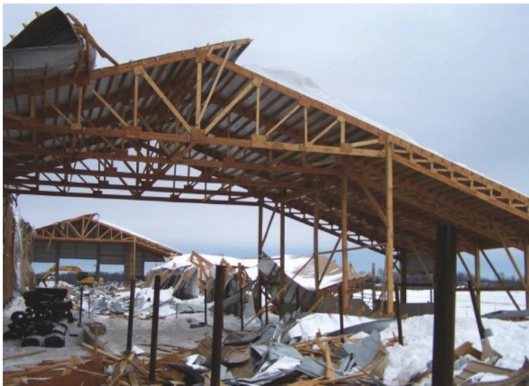
All but the endwalls and a middle section of this non-engineered building failed when columns buckled under, again, the first snow load. Subsequent calculations showed columns with a near-zero axial design load capacity.
