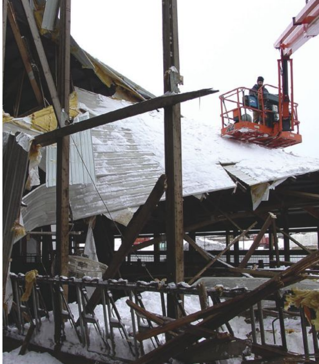
Workers remove roof sections that collapsed due to improperly braced trusses.
