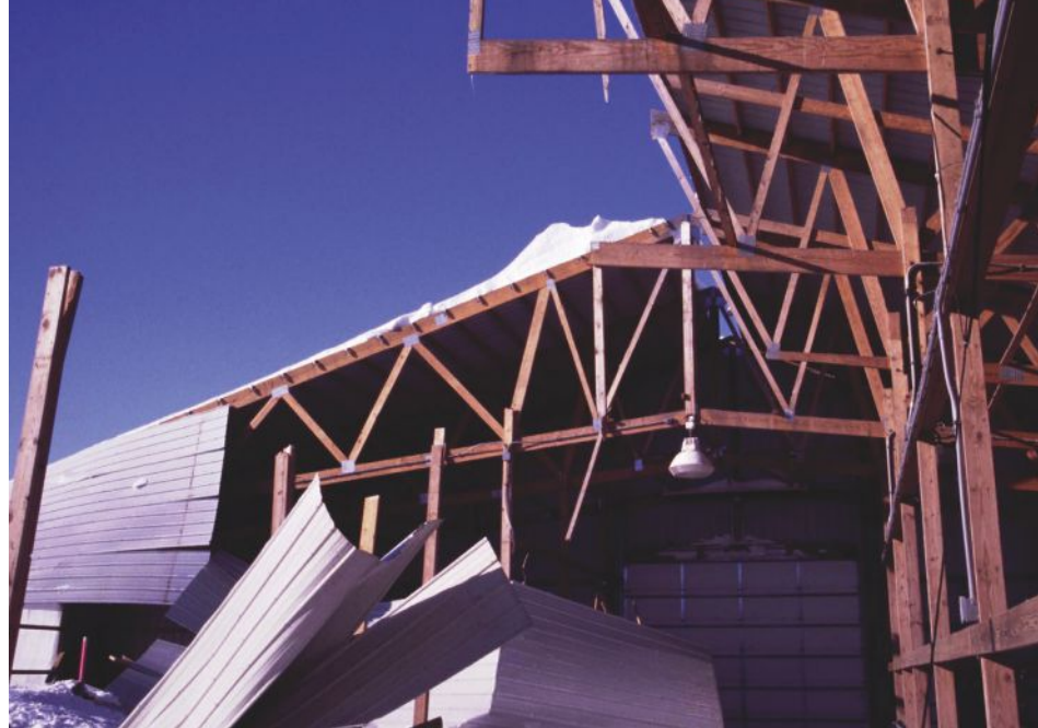
A non-engineered building that failed when truss webs buckled under the first snow load.
