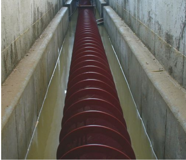
Sand settling lane with a collecting auger.
